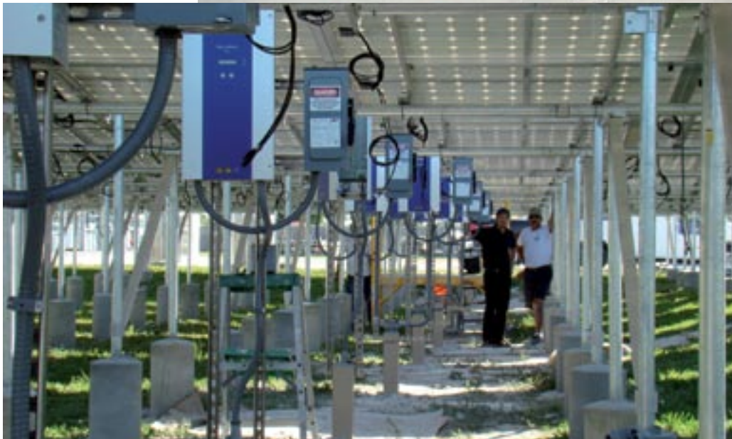
The largest pole-mounted solar power plant in Florida – of course with solar inverters made by KACO.
