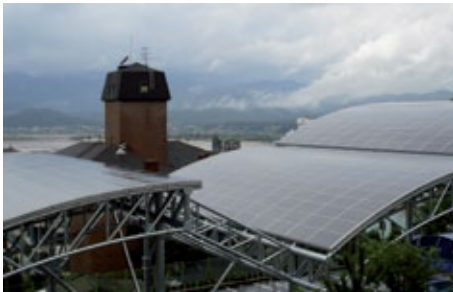
Kangwon, Korea Plant capacity: 120 kW
