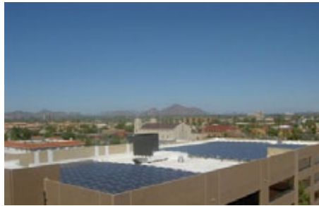
Health Care Cost Containment Building Phoenix, AZ, Plant capacity: 100 kW
