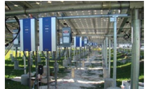
Florida Keys Electric Cooperative Marathon, FL, Plant capacity: 96 kW
